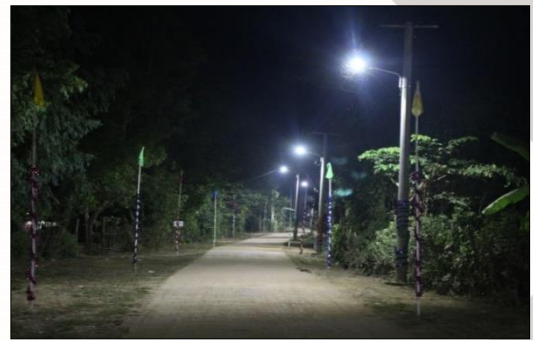
Installation of Village Road Electric Line in Byut Kalay Village, Dike-U Township, Bago Region
