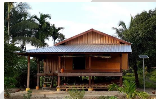
Installation of Solar Home System in Ywar Thit Village, Boke Pyin Township, Tanintharyi Region
