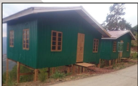
Construction of Rural House in Kyin Myar Village, Tedim Township, Chin State
