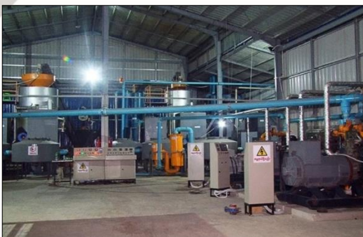
Installation of Biomass Electric Distribution System in Bi Tut Village, Laputta Township, Ayayarwaddy Region
