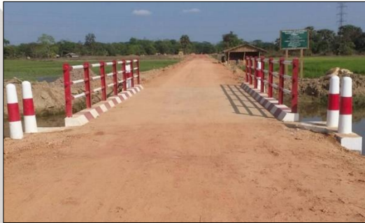
Construction of Farm Bridge in Thar Yar Kone Village, Tike Gyi Township, Yangon Region
