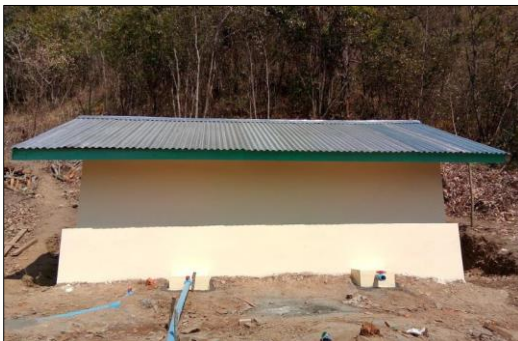
Implementation of Deep Tube Well in Latt Man (North) Village, Bu Ta Lin Township, Sagaing Region
