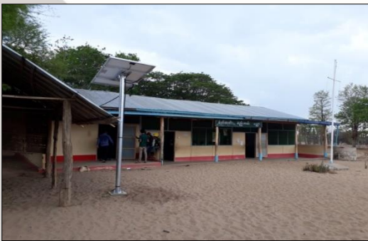
Installation of School Solar System in Tal Zar Village, Saytoattara Township, Magway Region
