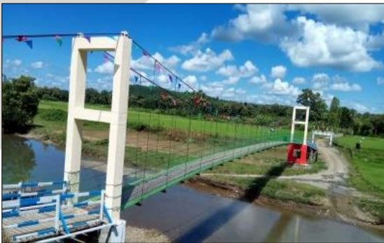
Construction of the Suspension Bridge in Kyat Wa Village, Min Don Township, Magway Region
