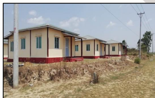
Construction of Rural House in Nyo Yaung Village, Sittwe Township, Rakhine State
