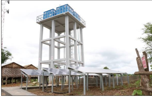
Construction of Water Supply Activities in Aye Chan Thar Village, Nya Pyi Taw
