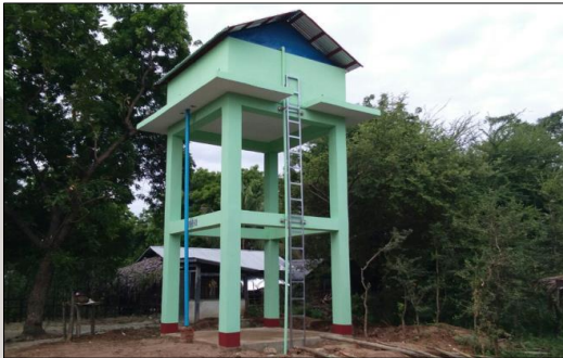
Water Tank in Tawma Village, Myaing Township, Mgway Region
